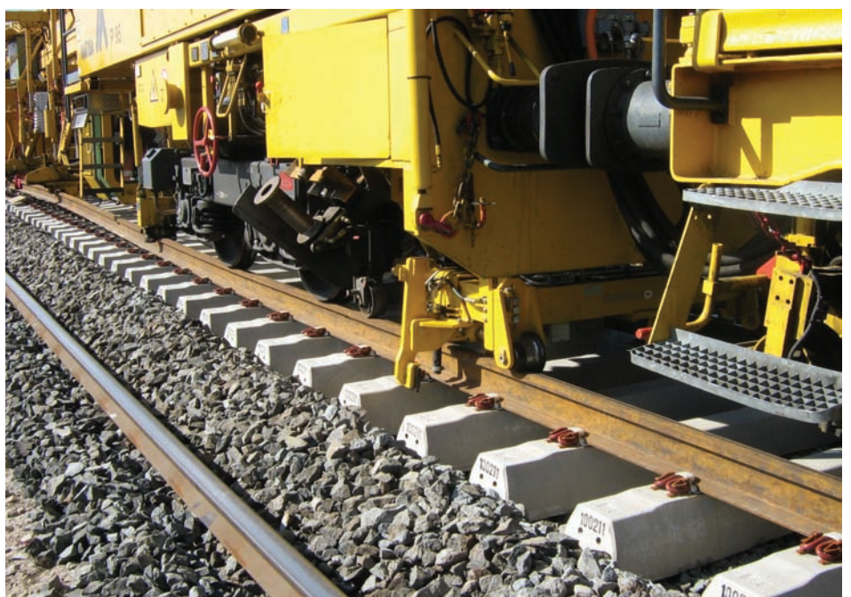
Clips correctly installed
